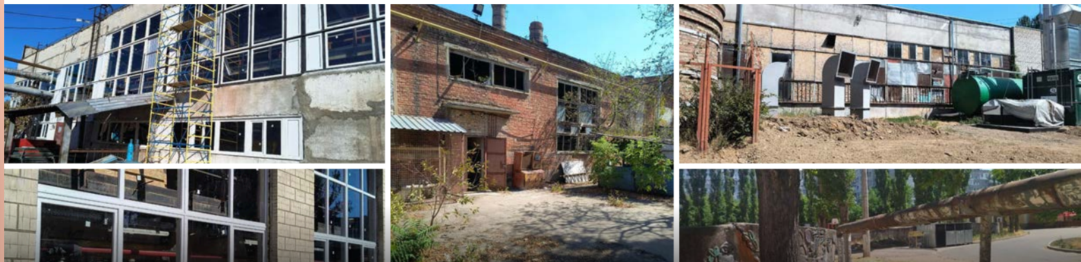
Several boiler rooms in the Mykolaiv region were damaged by direct hits and explosions. All damaged structures will be replaced as part of the project. Bottom right: thermal insulation in Mykolaiv, which is also planned to be replaced.
